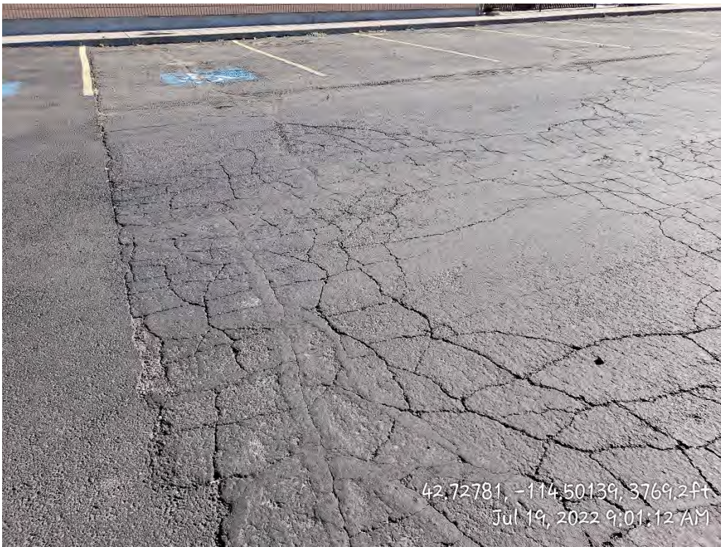
South of Building – Block and Alligator Cracking
