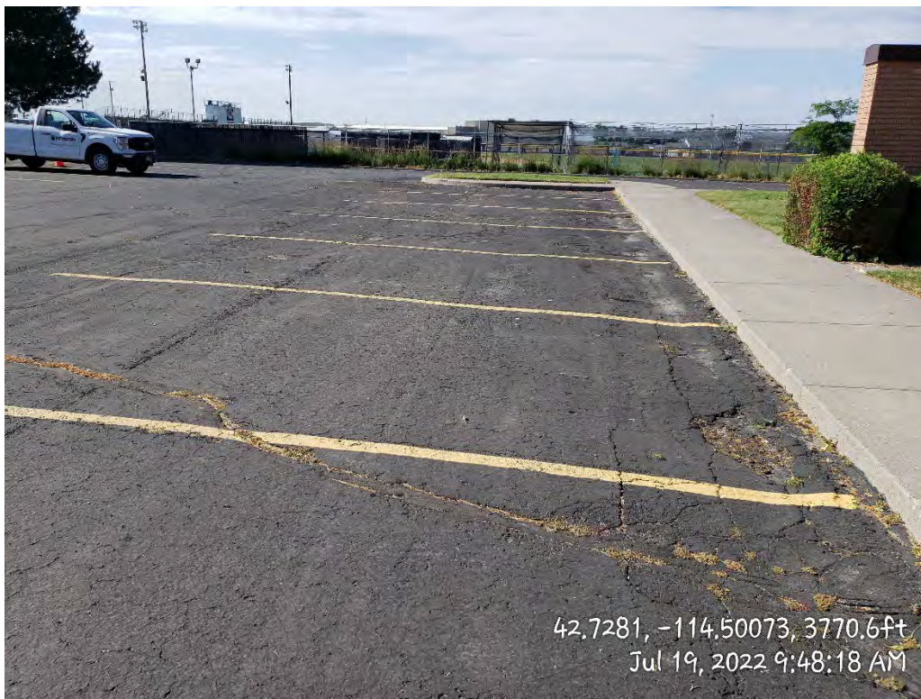
East of Building – Alligator Cracking, Raveling, and Rutting Adjacent to Curbing
