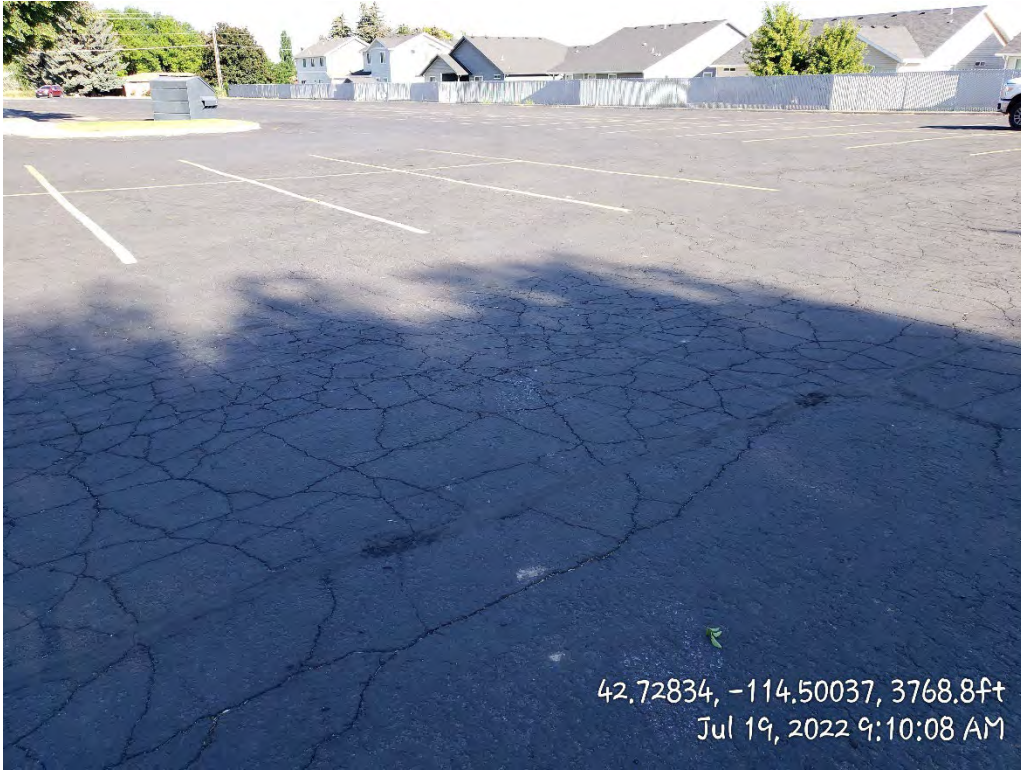
East Lot – Block and Alligator Cracking
