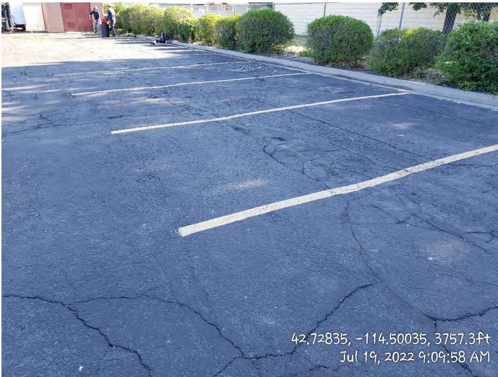
East Lot – Transverse, Longitudinal, and Block Cracking
