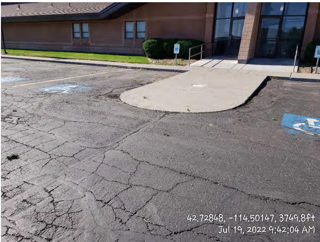
North of Building – Block and Alligator Cracking with Rutting Adjacent to Curb
