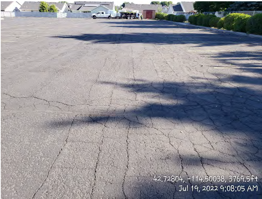
East Lot – Transverse, Longitudinal, Block, and Alligator Cracking
