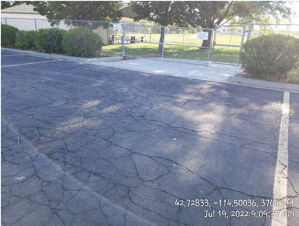
East Lot – Block and Alligator Cracking
