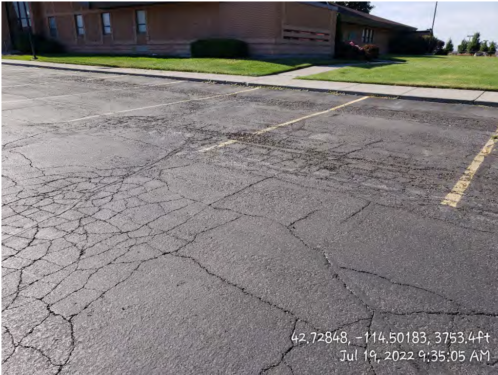
North Lot – Block and Alligator Cracking with Raveling
