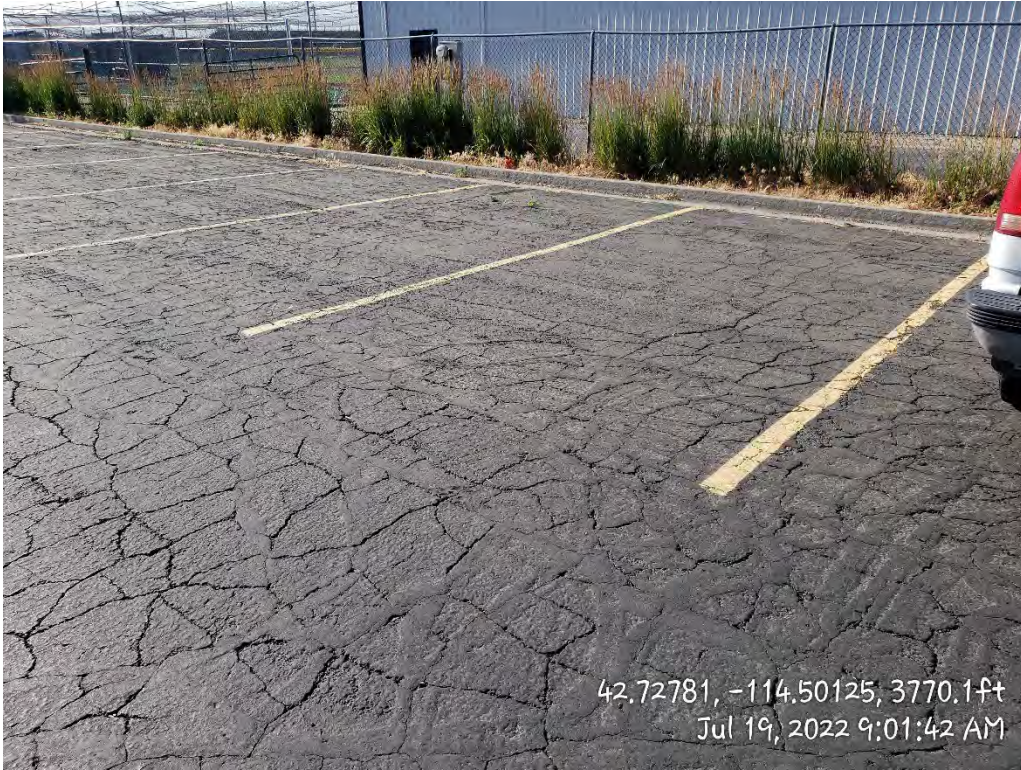
South of Building – Alligator Cracking
