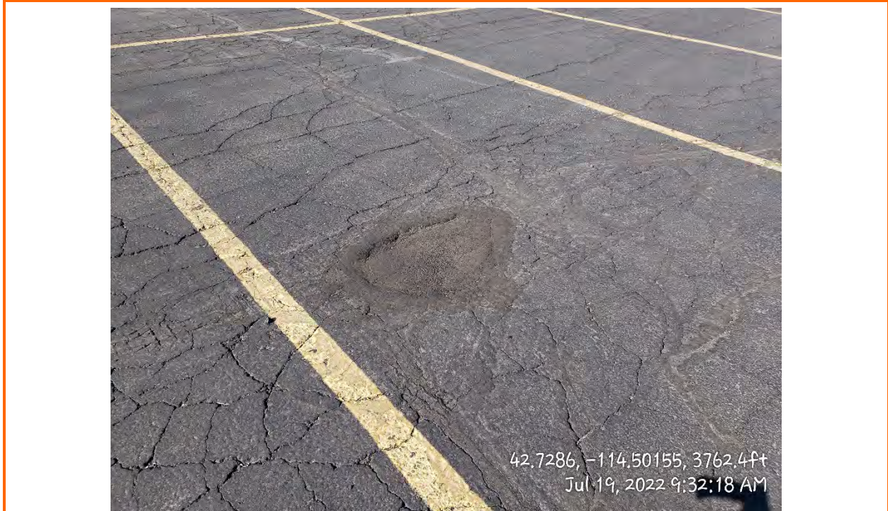
North Lot – Block and Alligator Cracking with Pothole
