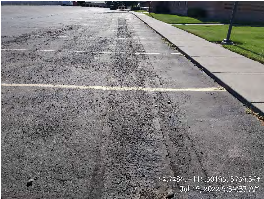
North Lot –Patch with Raveling
