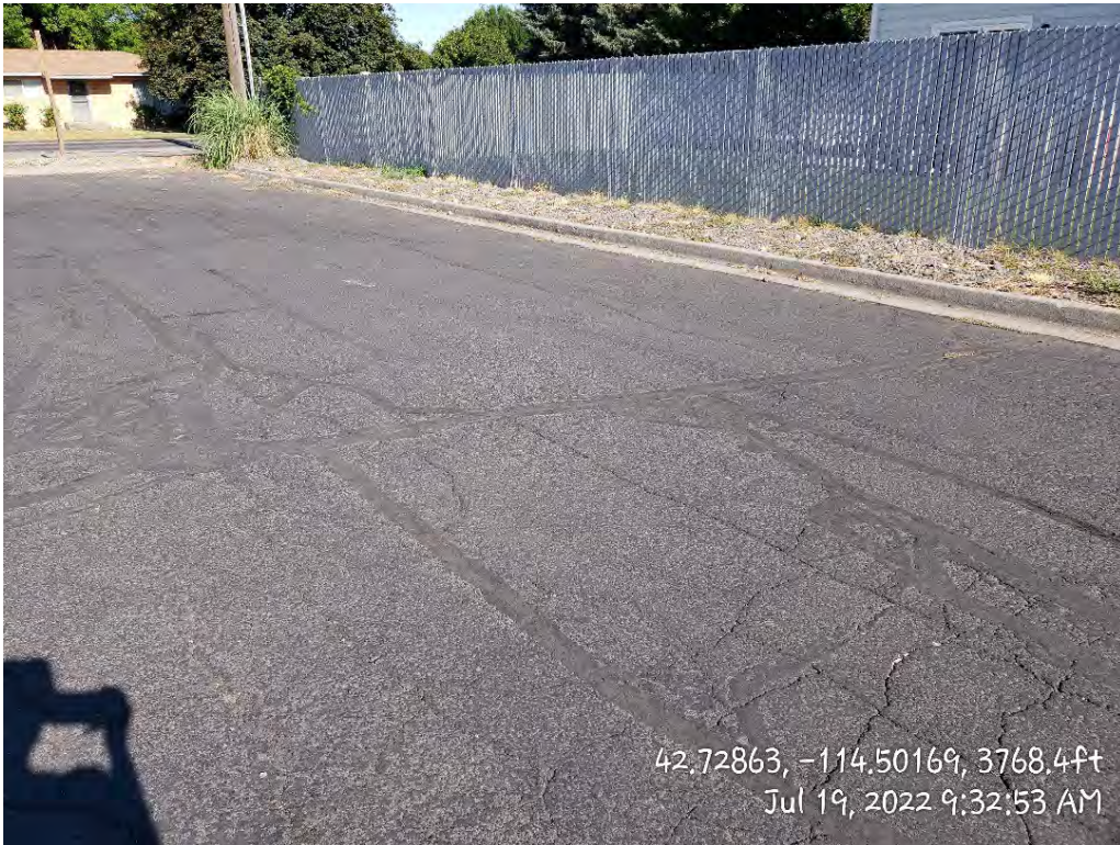
North Lot – Transverse, Longitudinal, and Block Cracking, Some with Sealant
