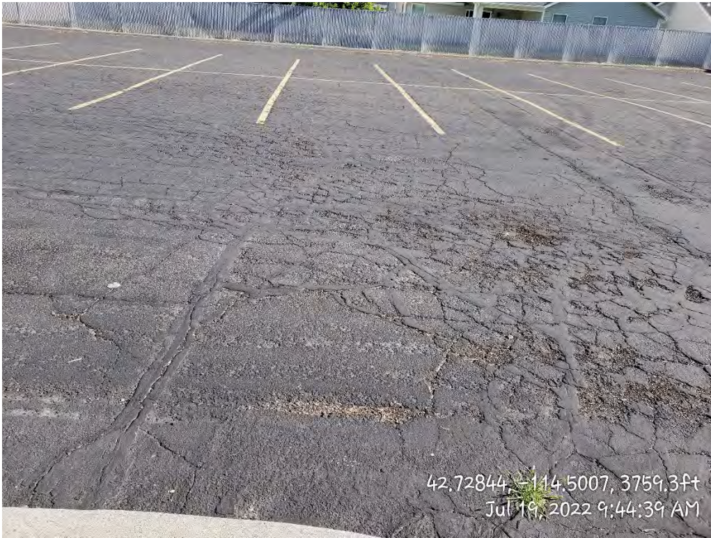
North Lot – Block and Alligator Cracking with Utility Patch
