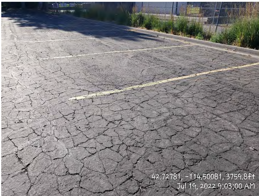
South of Building – Alligator Cracking
