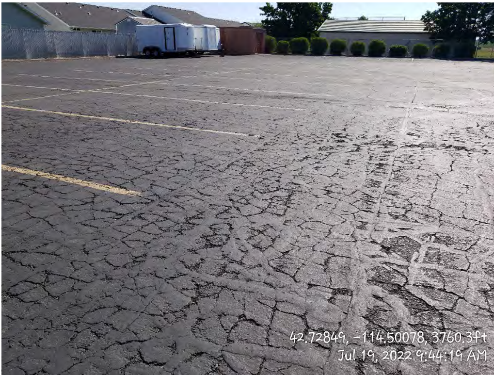
North Lot – Alligator Cracking
