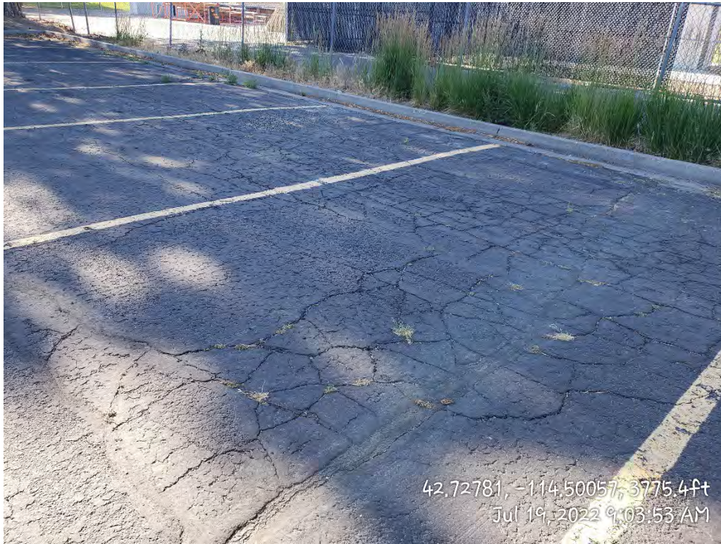
East of Building – Block and Alligator Cracking
