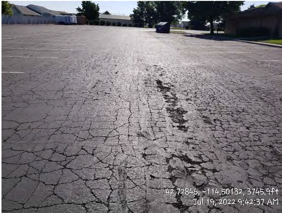
North Lot – Alligator Cracking and Raveling
