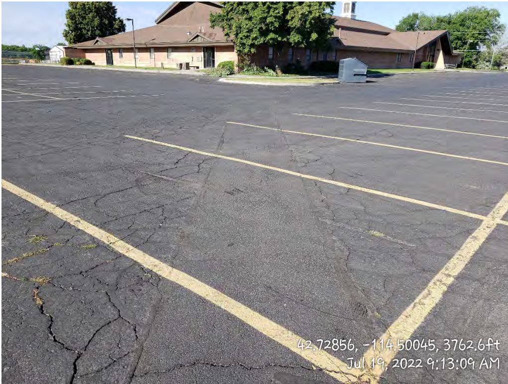
East Lot – Utility Patch with Cracking
