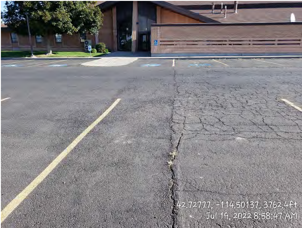
South of Building – Transition from Distressed to Less/Non-Distressed Pavement
