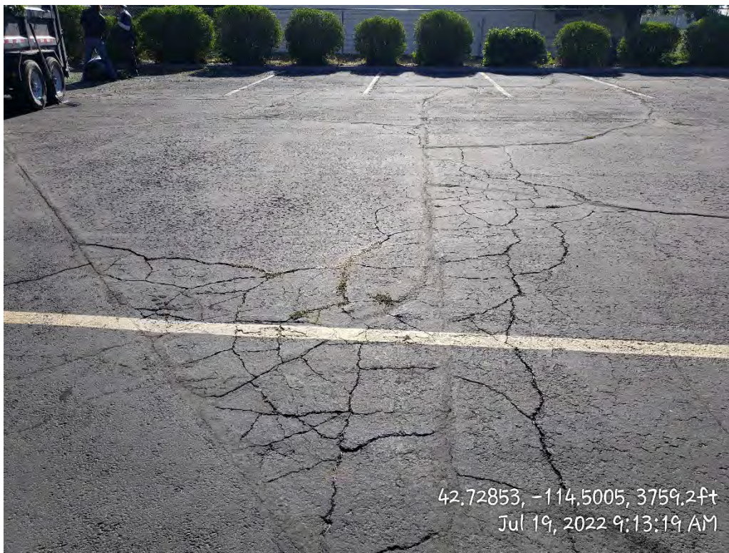
East Lot – Block and Alligator Cracking
