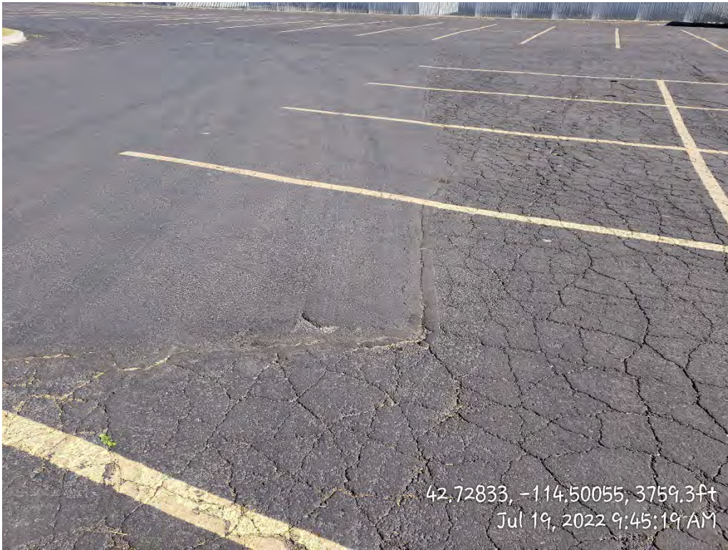
East Lot – Alligator Cracking with Repair Patch
