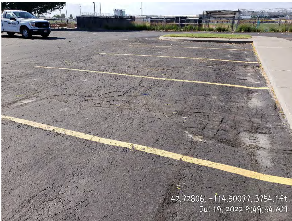
East of Building – Alligator Cracking and Rutting Adjacent to Curbing
