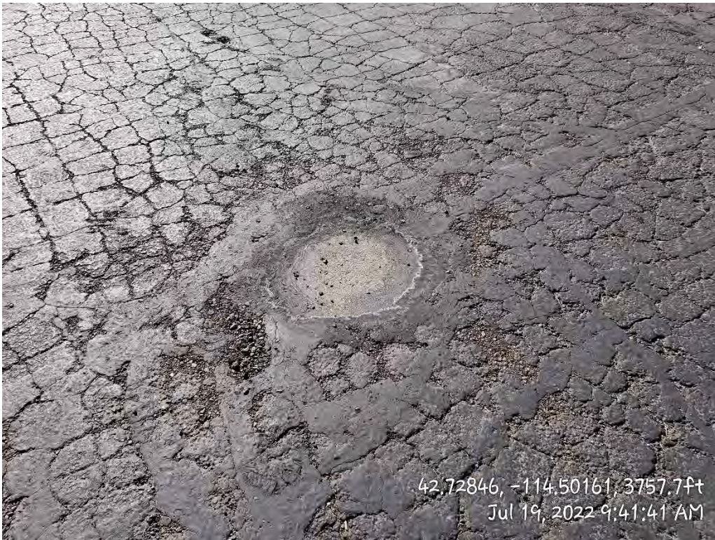
North Lot – Alligator Cracking and Raveling with Pothole
