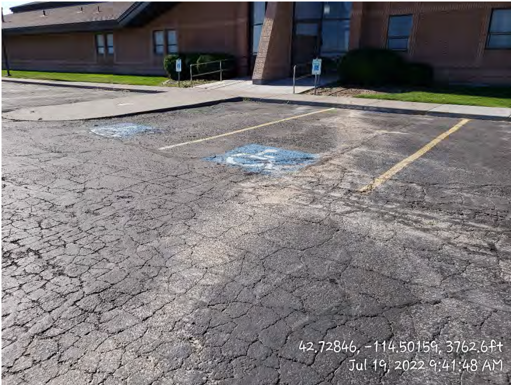
North of Building – Block and Alligator Cracking with Rutting Adjacent to Curb
