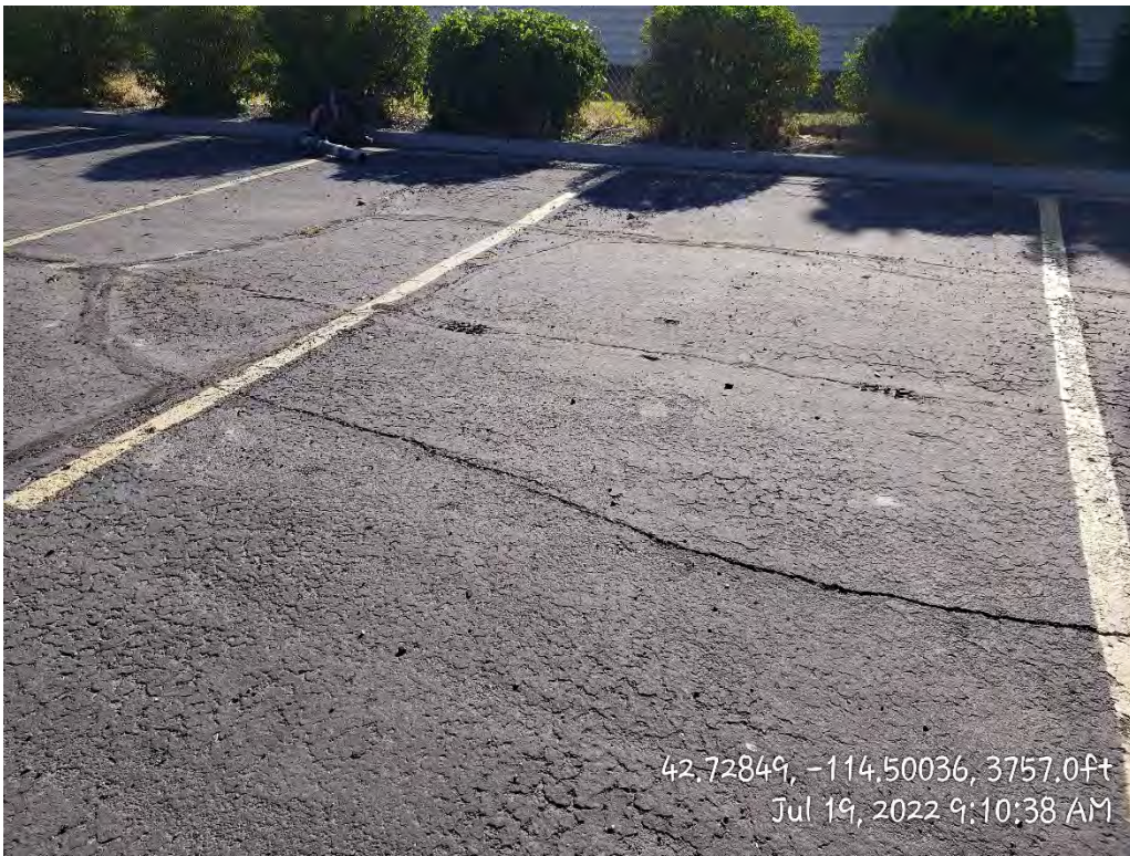
East Lot – Transverse and Longitudinal Cracking with Raveling
