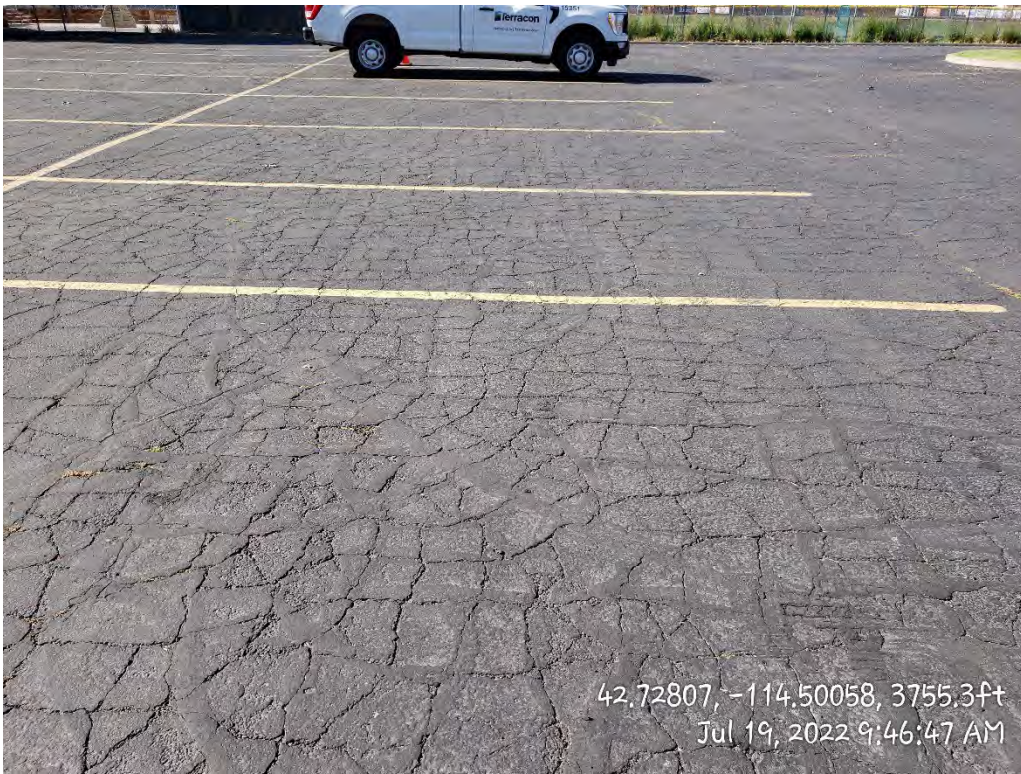
East Lot – Alligator Cracking
