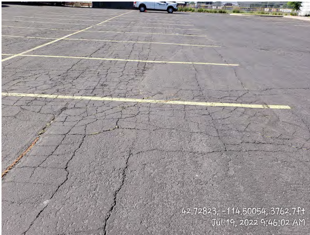
East Lot – Block and Alligator Cracking
