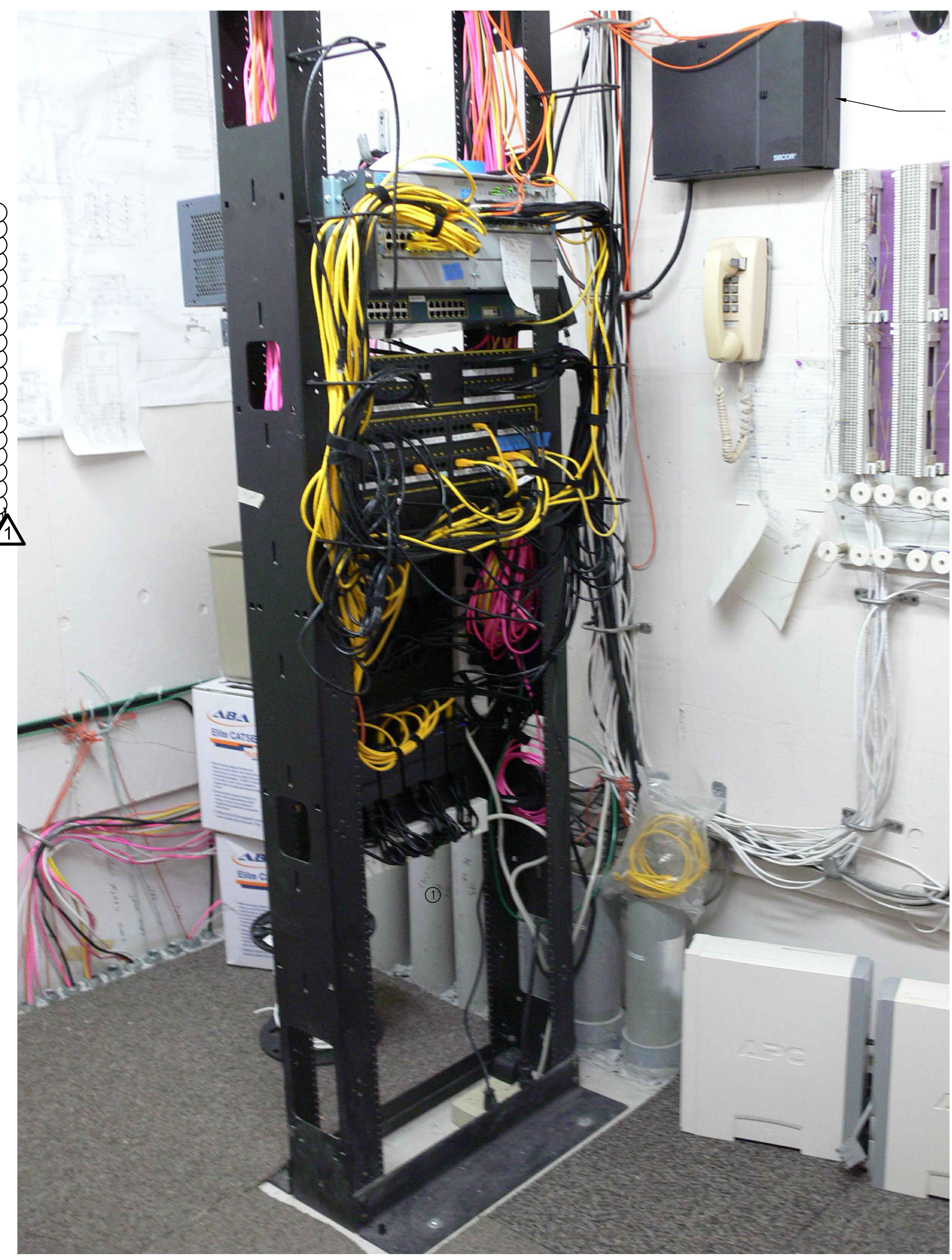
ROOM 114 DATA RACK (ALTERNATE #4)
